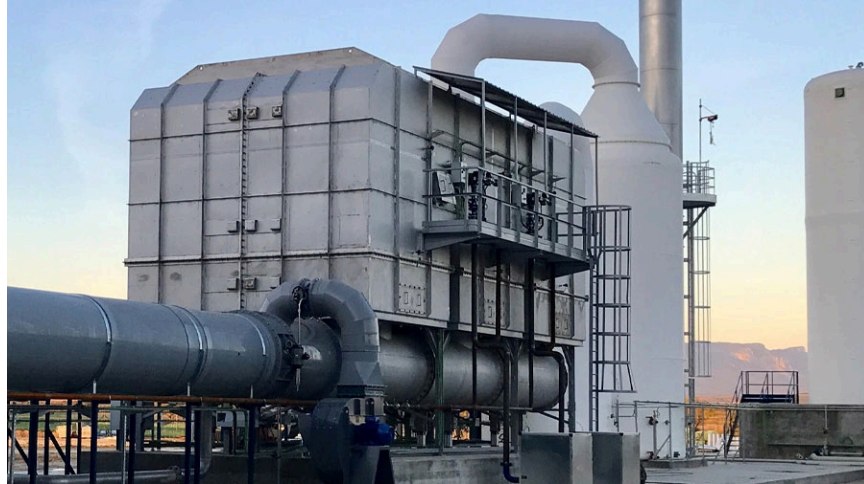
Figura 1.14: Depurador o scrubber . (Scrubbers for Air Pollution Control: What Are They?, 2019)
