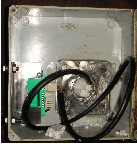
(a) Interior view of the sensor node container
