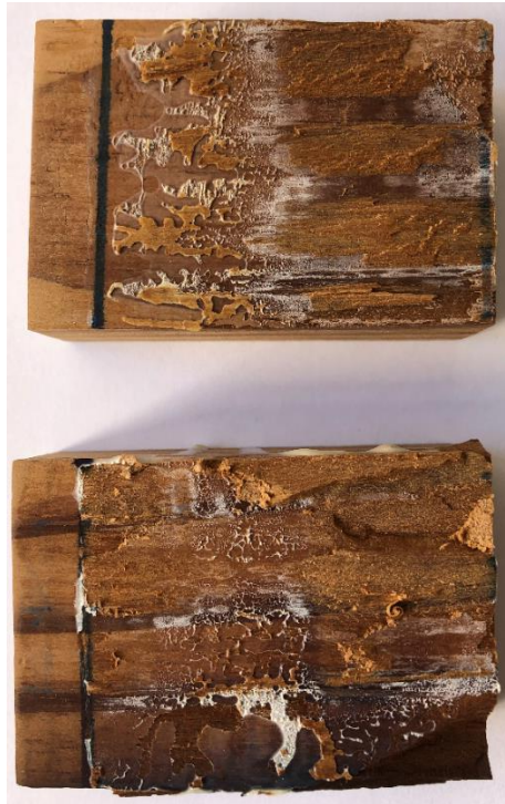
Figure 4.48 EPI adhesive failure on modified P. taeda . Adhesive remained at the surface, evidencing penetration problems
