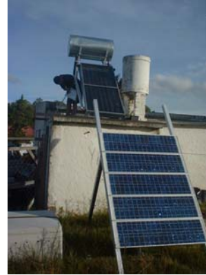
Fig. 9. Quebracho, Uruguay. Solar water heater system and PV system.
