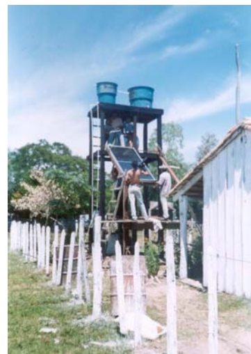
Fig 6. Punta Diamante, Paraguay. Solar water heaters with insulated tank at the school
