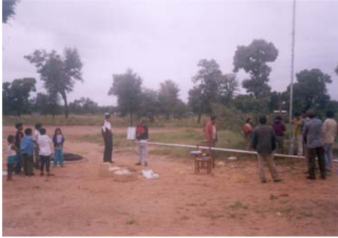
Fig 7. Yacac Vash, Paraguay. Instalation of public lighting with the colaboration of community people.
